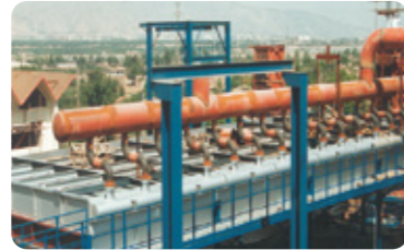
Continuous Reforming Unit of Lanzhou Refinery
