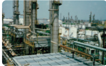
Air cooler of Shanghai Jinshan Petrochemical Aromatics Plant
