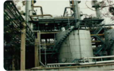
Air cooler of Yanshan Petrochemical p-xylene plant
