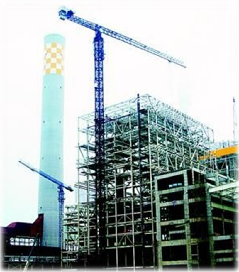
Puqi Power Plant 2X1000MW New Project, High Ash Time of Commission: Oct, 2012
