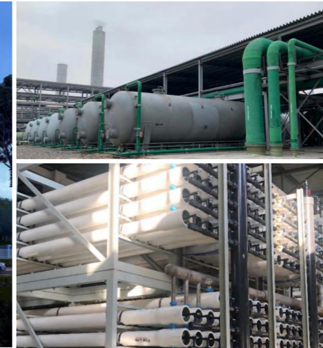
大型卧式砂滤 Large horizontal sand filter
