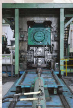
操作侧 Operation Side
