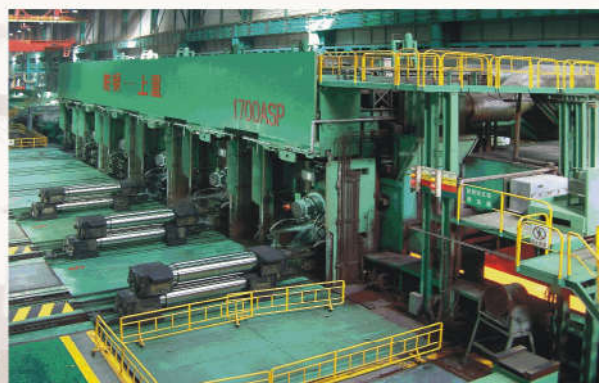
为济钢自主设计制造的1700mmASP热连轧机组 (精轧区) 1700mm ASP self-designed hot tandem rolling line finishing mill section for Jigang
